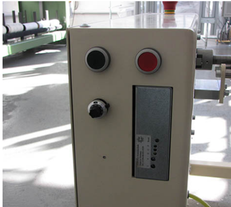
Bedienpanel Control panel
